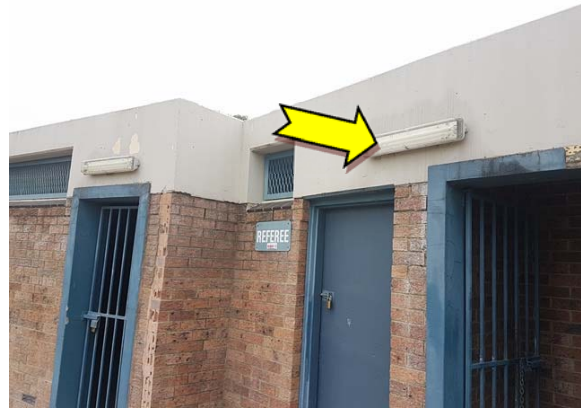
Photo 2. Exterior, throughout, single tubed fluorescent light fitting – suspected non PCB-containing capacitors.
