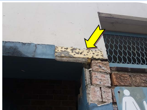
Photo 6. Exterior, upper level walls – suspected lead-containing yellow lower paint systems.
