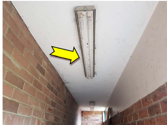
Photo 4. Interior, south-east elevation, store room, double tubed fluorescent light fittings – suspected PCB-containing capacitors.
