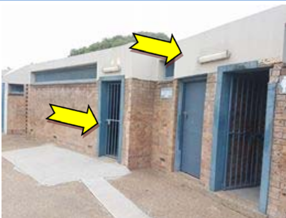
Photo 5. Exterior, upper level walls, window and door frames – suspected lead-containing beige and blue upper coloured paint systems.
