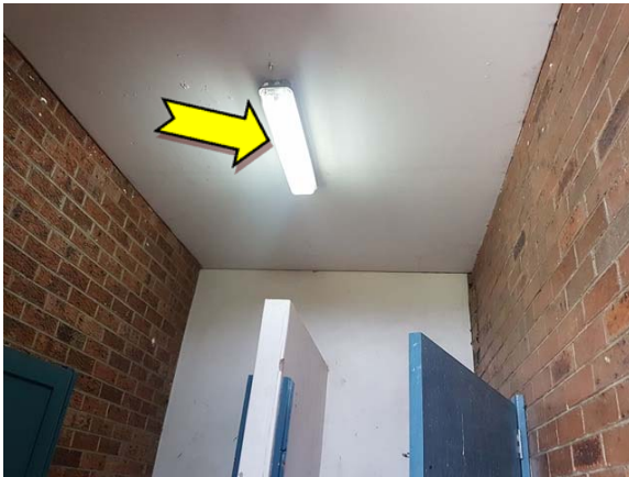
Photo 3. Interior, throughout, single tubed fluorescent light fitting – suspected non PCB-containing capacitors.
